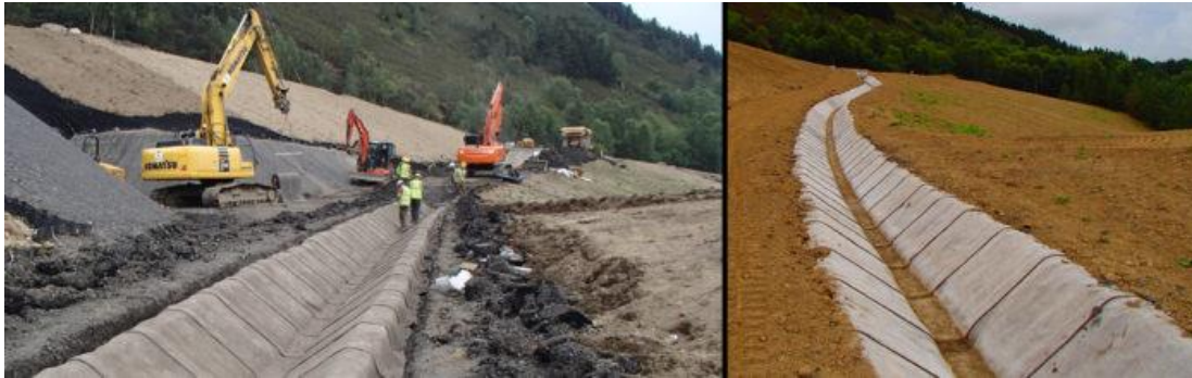
Figure 3. Water diversion at a mine in Ireland with lined channel (left). At HVC we lined one of our ditches with impermeable till or used pipelins where we crossed exposed bedrock with toppling potential structures (right)
